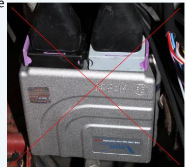
Picture 2c: ECU incorrectly fitted
